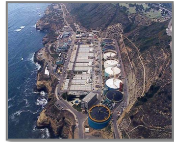
Savings at the Point Loma Plant. Savings at the Point Loma Plant played an important role in establishing reuse targets. The land available at Point Loma Site is constrained, and any upgrades incur high costs.
