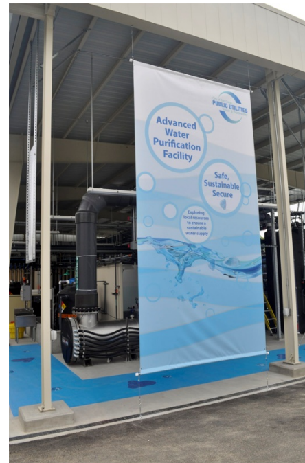
The Demonstration Facility was installed and operated to produce and test purified water.
