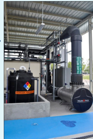
Step 3: Ultraviolet Disinfection/Advanced Oxidation
