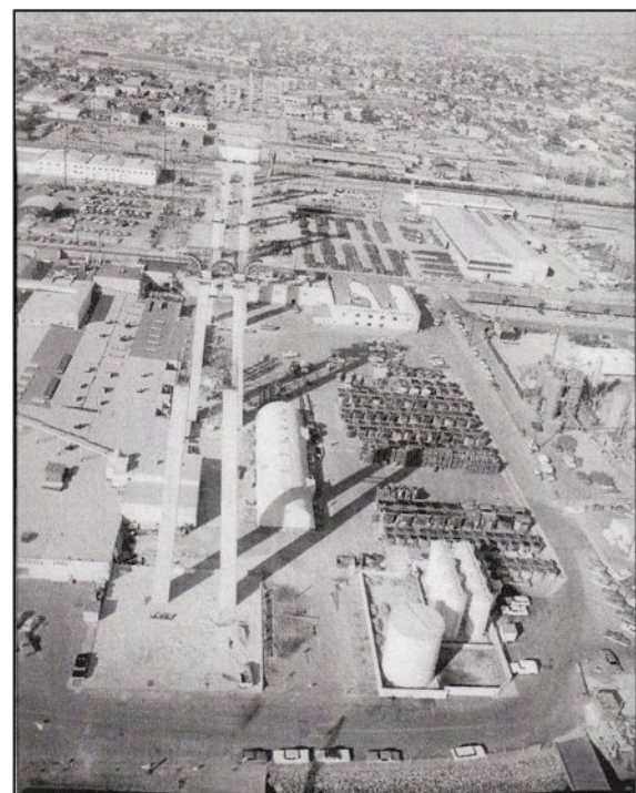
Plate 14. Coronado Bridge construction over Barrio Logan in 1969, facing east. Courtesy of SDHS (#UT-85-08564-2)
